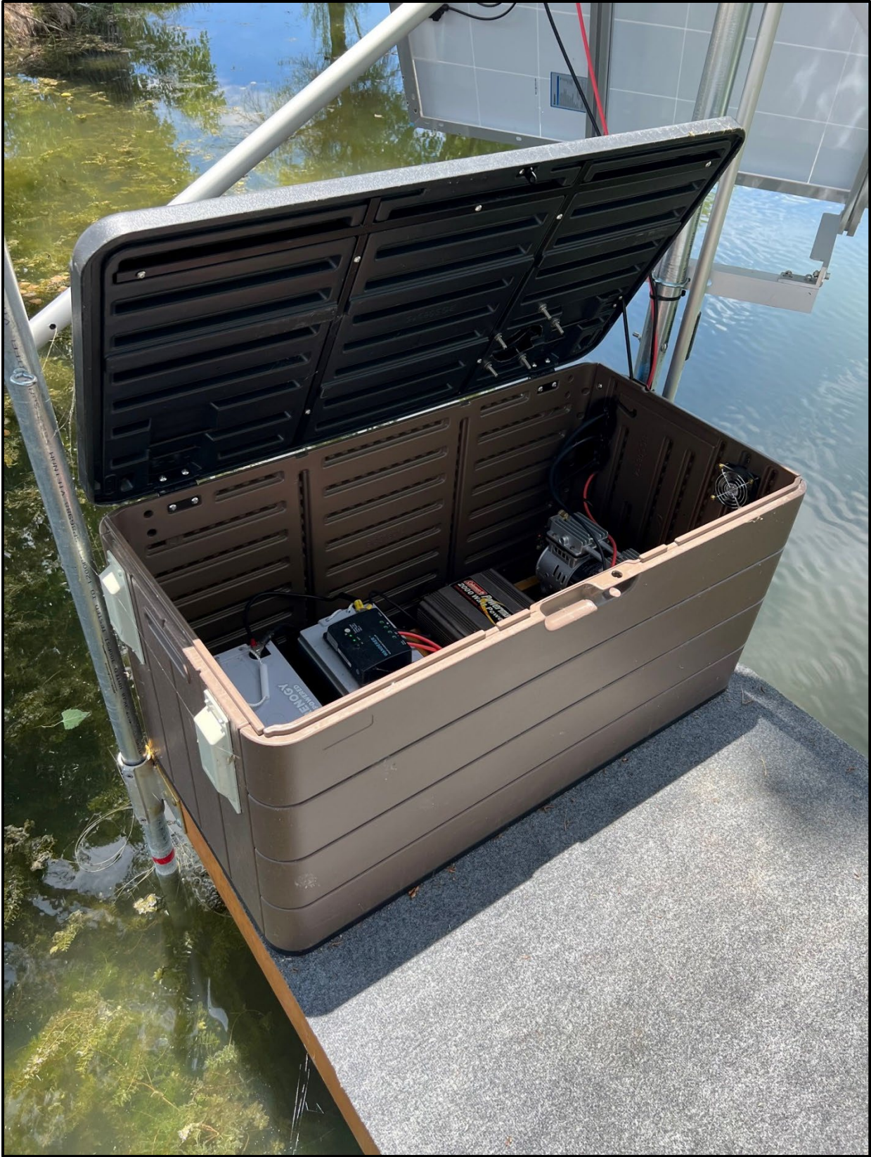
Solar panels charge batteries to store power for aeration pump.
